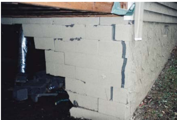
This is what happens to a block wall when the openings do not meet code and hydrostatic pressure is not equalized.
