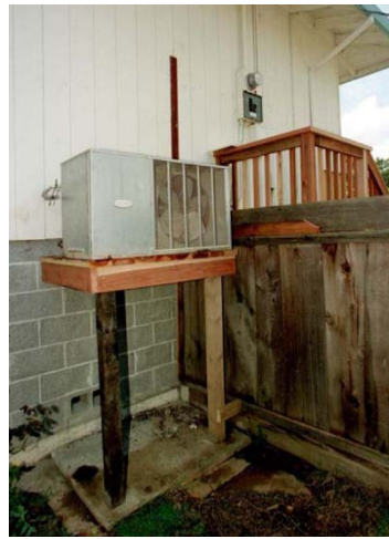
This house has an elevated air conditioning compressor and electric meter.
