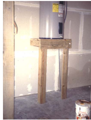
The owner replaced a flood damaged water heater with a shorter one and elevated it.
