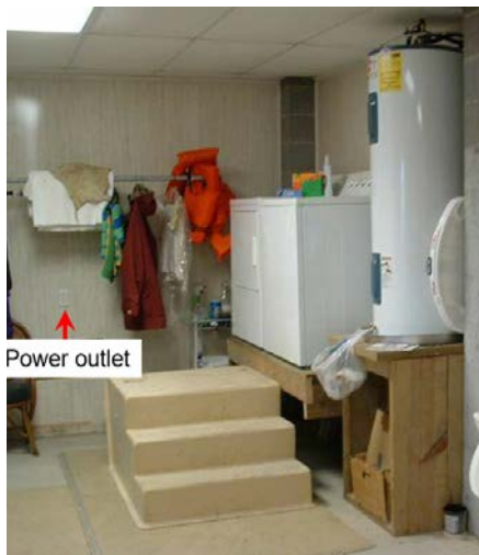
The washer, dryer, and water heater were elevated in this wet floodproofed garage.
