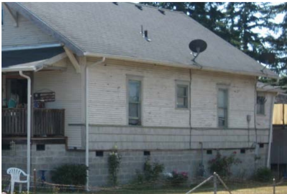
This is an example of an improperly elevated building. The openings are too high to relieve hydrostatic pressure.
