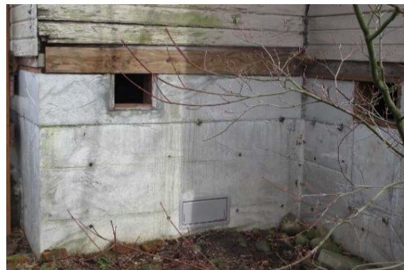
This building in Bucoda was retrofitted with flood vents near the ground that automatically open to let water in.
